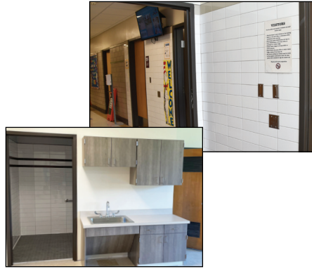
Significant work was completed at South Side (above), including new tiling in the hallways, updated bathrooms and ADA-compliant classroom doors.
